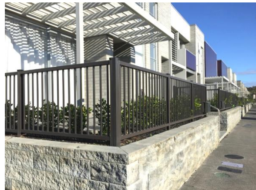
Figure 2. Moduline safety fence installed in concrete pile footings behind a retaining wall.
